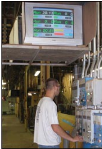
A video screen near the chrome line provides visual confirmation of process conditions, including time left in tank and other variables.
